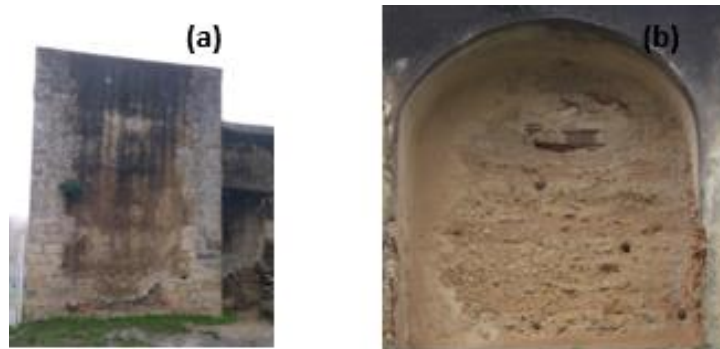
Figure 5 – Gil Vicente's School: (a) small tower with stone masonry corners and rammed earth and (b) rammed earth section of the Wall
