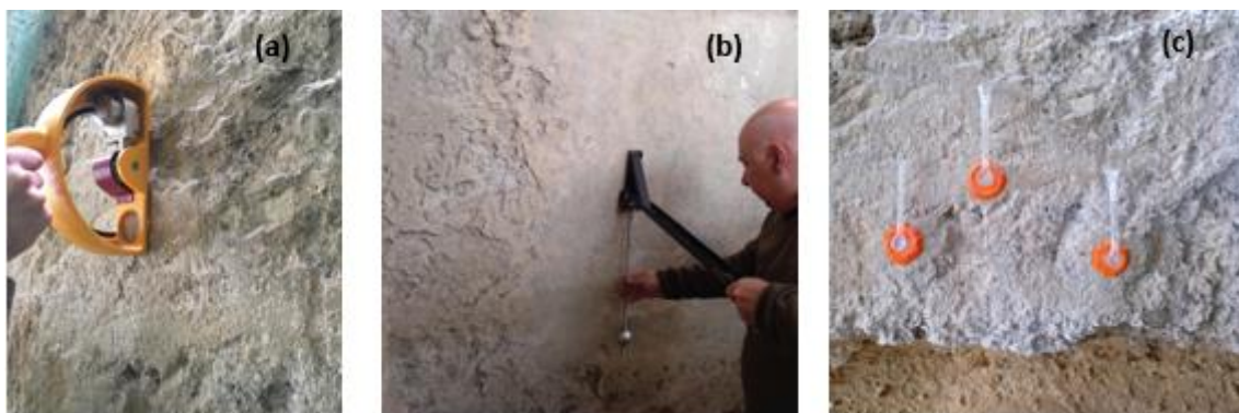
Figure 9 – In situ tests: (a) Pendular sclerometer in Bragança Terraces Residence wall section facing south; (b) Sphere impact test at a wall facing East inside Jogo da Pêla Tower and (c) Karsten tubes test at a wall section facing East at Bragança Terraces Residence
