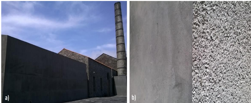
Figure 2 – Building technique similar to the Brita Lavada , applied for reinforced concrete (a); two different types of surface in detail, smooth and rough (b).
