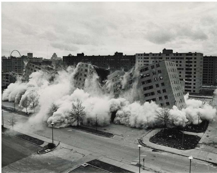
Demolition of Pruitt-Igoe, 1972, U.S. Department of Housing and Urban Development Office of Policy Development and Research.
