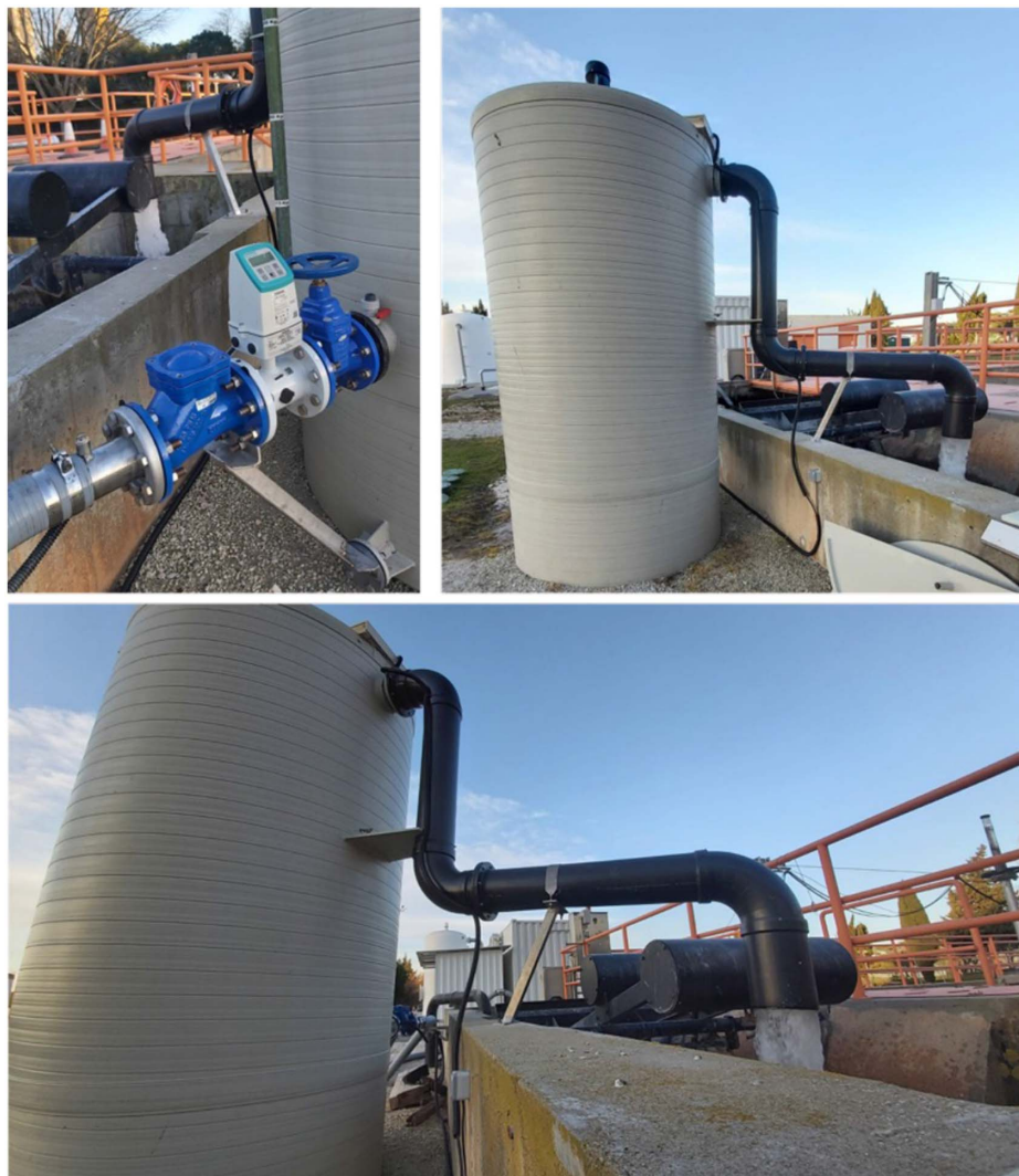
Fig. 1. Pilot installation at the wastewater treatment plant.
