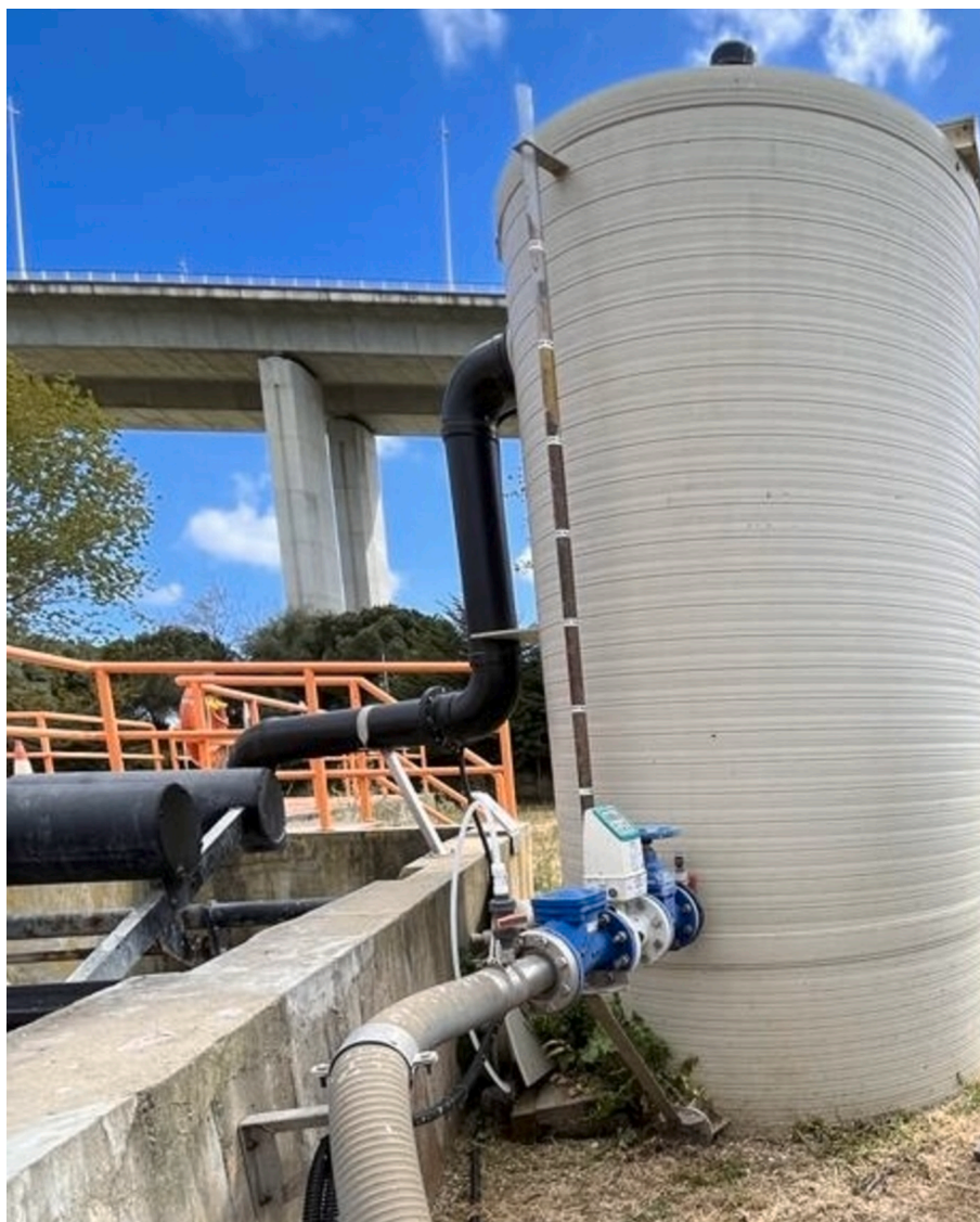
Fig. 1. Pilot-scale installation set-up.
